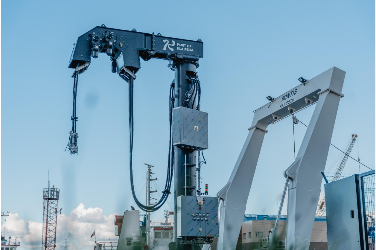
Figure 2. Onshore power supply (OPS) station for Ro-Ro ferries
